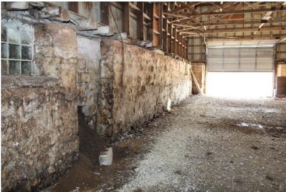
The floor was removed which altered the lateral system. The barn was leaning and in danger of collapse.
