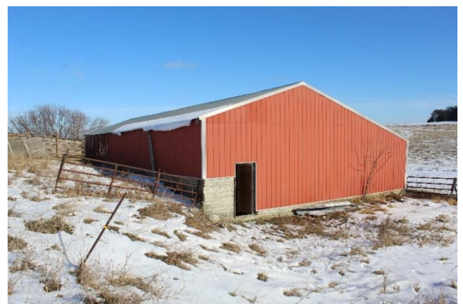
Unbalance soil load caused the standard pole shed to lean
