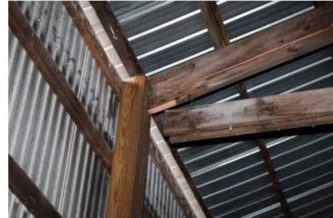
The bottom chord of the truss came loose. Identically made trusses were a hazard.
