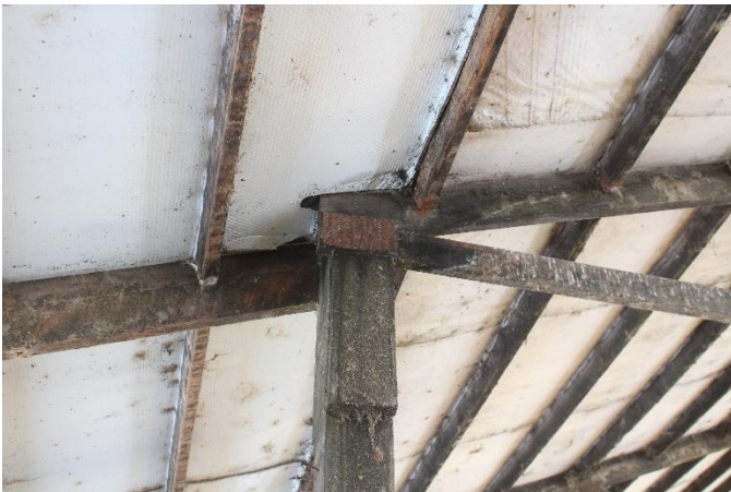
The barn had weak connections beyond the collapse.
