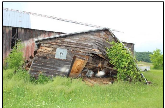
The building had not been used in a very long time. Collapse was a predictable event.
