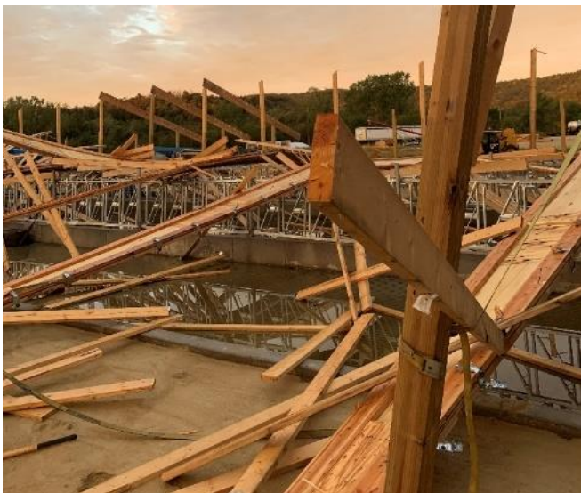
The freestall barn collapsed while under construction.
