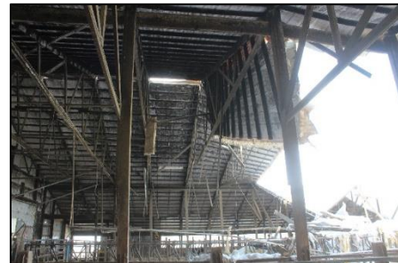
2/3 rd of the roof structure collapsed. The remaining roof structure was unreliable.
