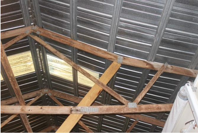
The truss failed at the top chord splice location.
