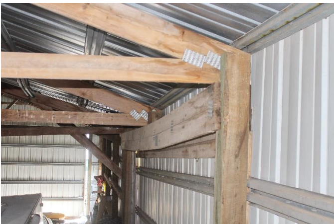
The beam above the door was deflecting.
